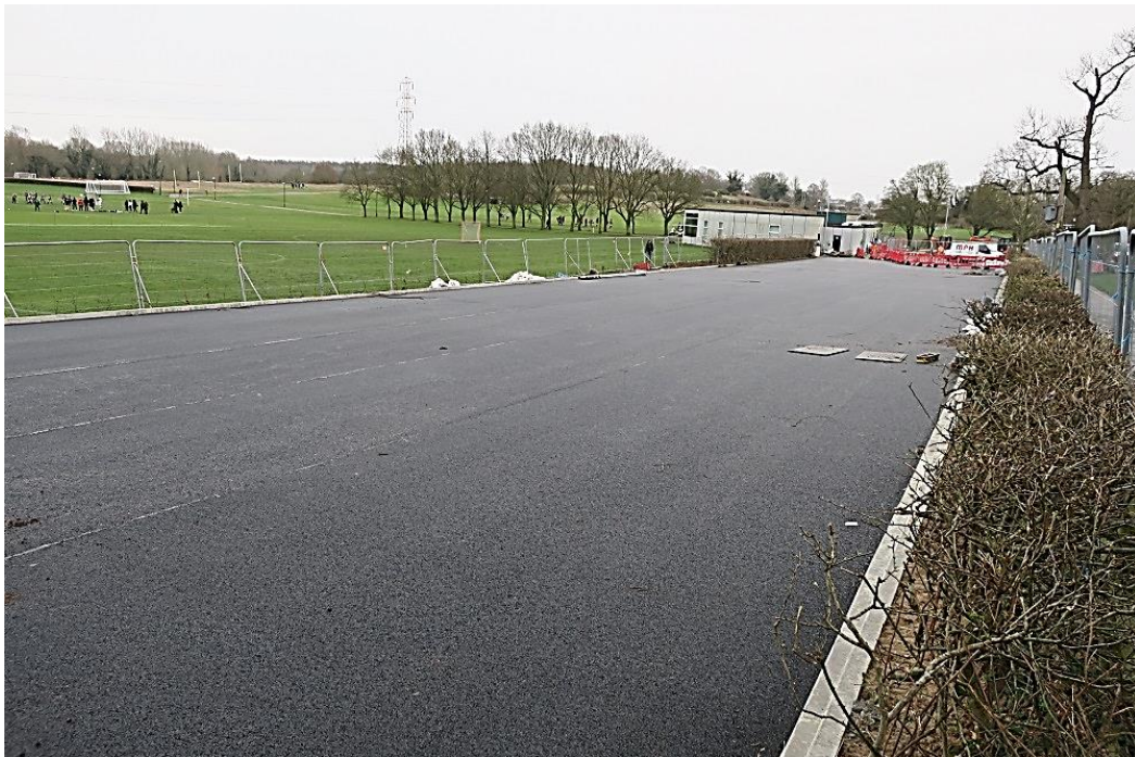
Yare Valley Green Space disappears under impermeable asphalt. Run-off?
